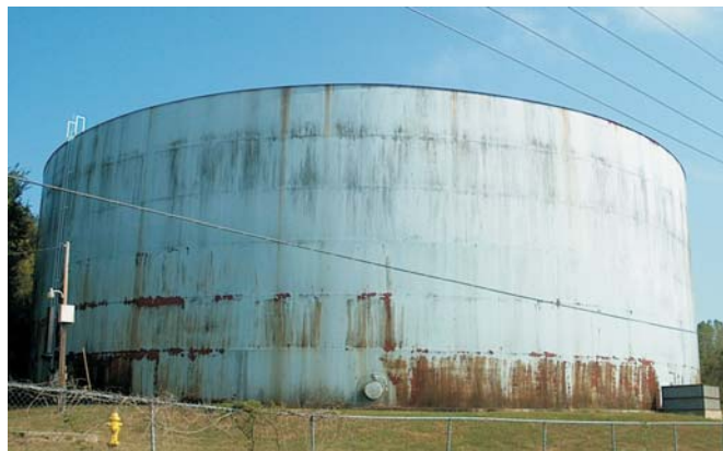
Bowlin Road Ground Storage Tank
